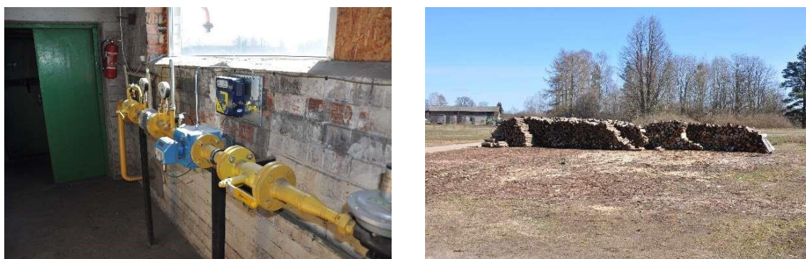
Figure 5.3.2. Fuels used in the Palsmane Village boiler house: natural gas and wood
